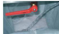
Clear water discharge
