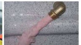
waste water entry
